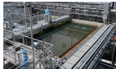
Wastewater treatment equipment installed at a plant
